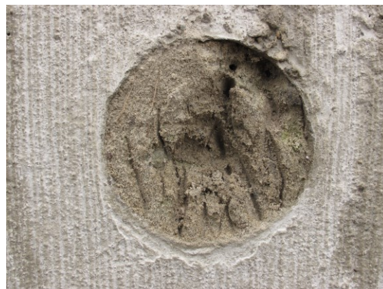
Nestingang in betonnen wand
